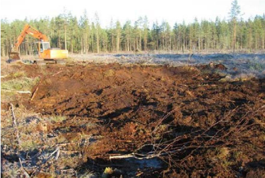
Figure 2. The view of an old ditch after blocking using an excavator at site ResB1.
