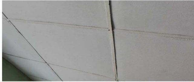
Figure 1. Some pictures of the physical condition of the classrooms
